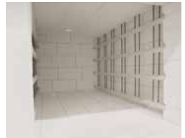
Protection grid in front of heating elements prevent against mechanical damages
